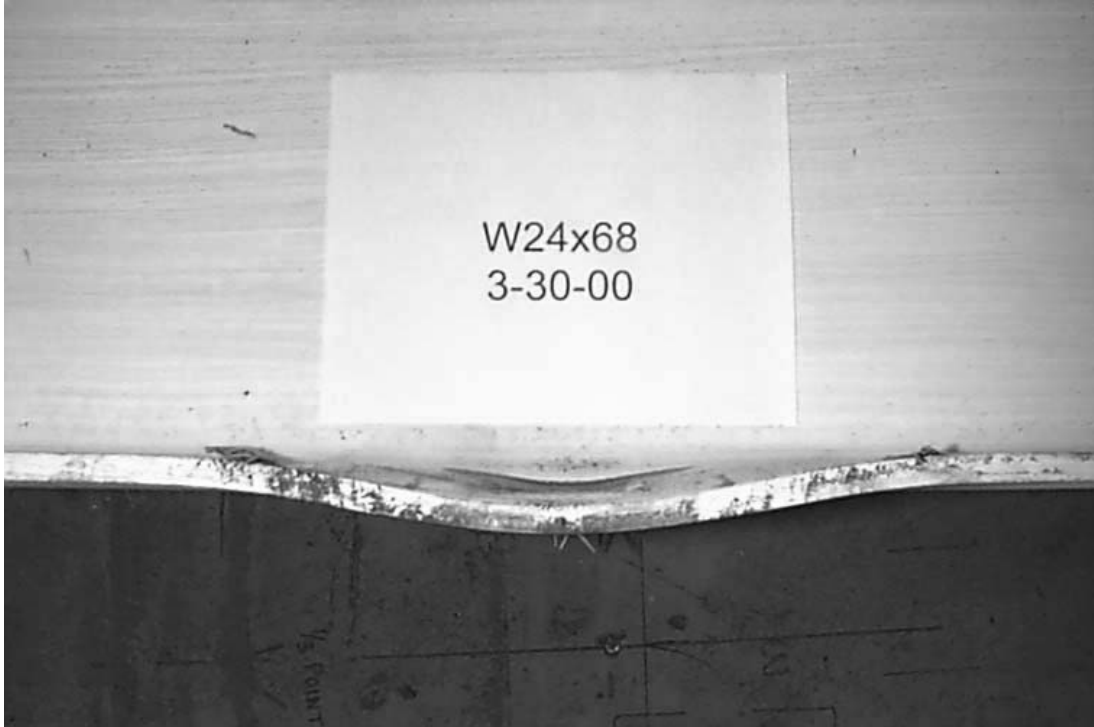
Figure 9. Bottom Flange Deformation
