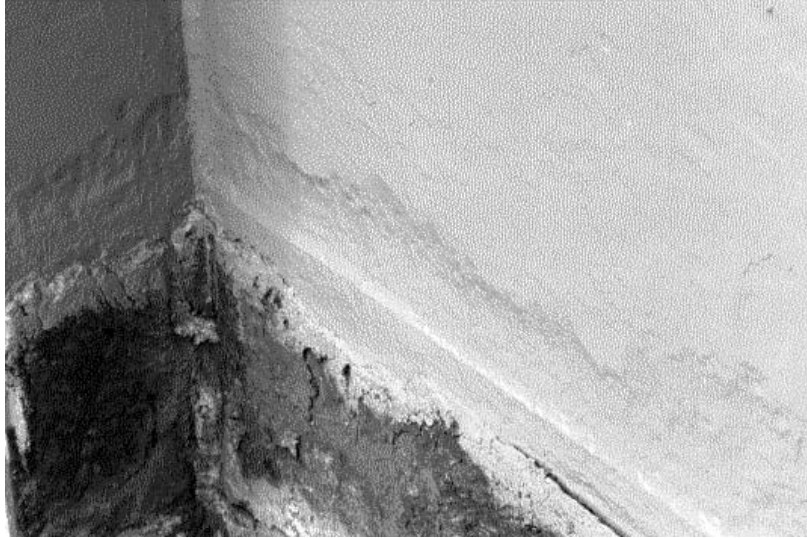
Figure 2. Corrosion at the bridge deck level.
