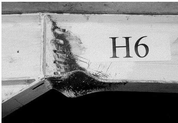
Fig. 4 View after failure of H6
