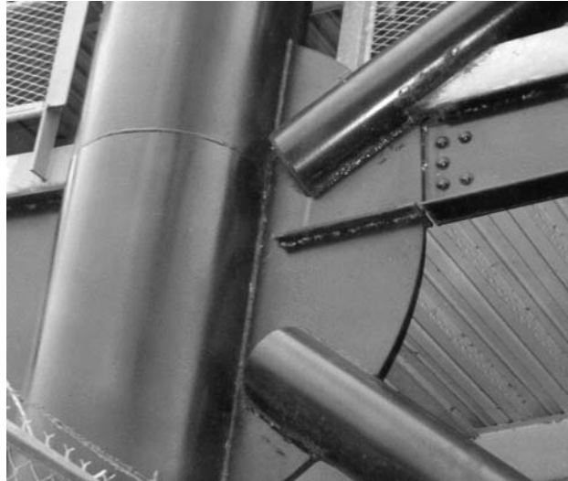
Figure 6. Photograph of Prototype Connection
