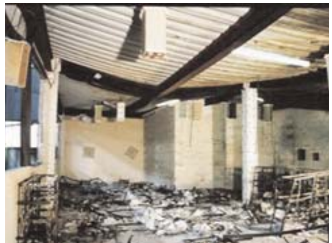
Fig. 6.4. Unprotected Steel Floor System After 1996 Cardington, U.K. Fire Test (Newman et al, 2000) (Photo courtesy of Corus Research Development & Technology)
