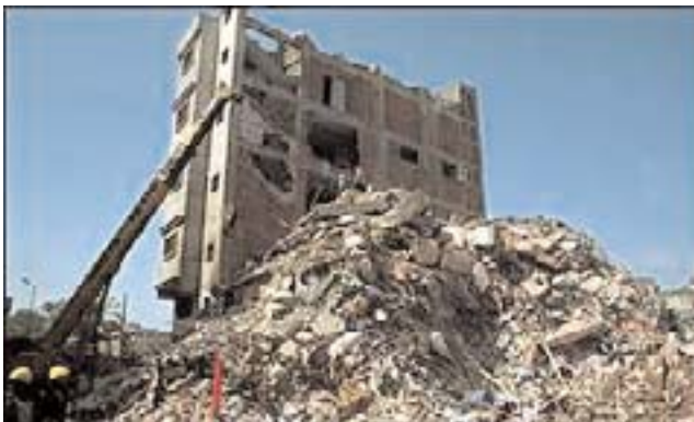
Fig. 7.2. Collapsed Textile Factory in Alexandria, Egypt (BBC New, 2000)
